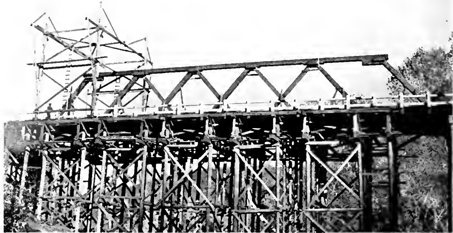
With falsework supporting deck and a traveling gantry new truss is being installed
